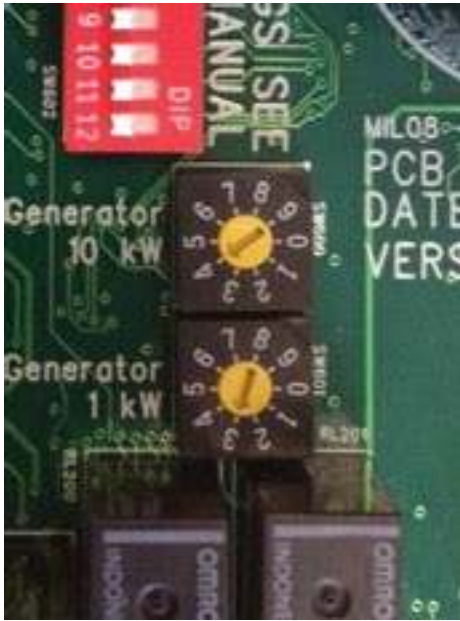
Figure 6 – Generator Power Rotary Switches
